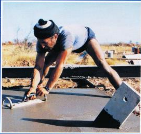
Above: Completing the concrete pour on a guy anchor block. Right: Tensioning steel guy ropes. Below: Erecting mast section.
