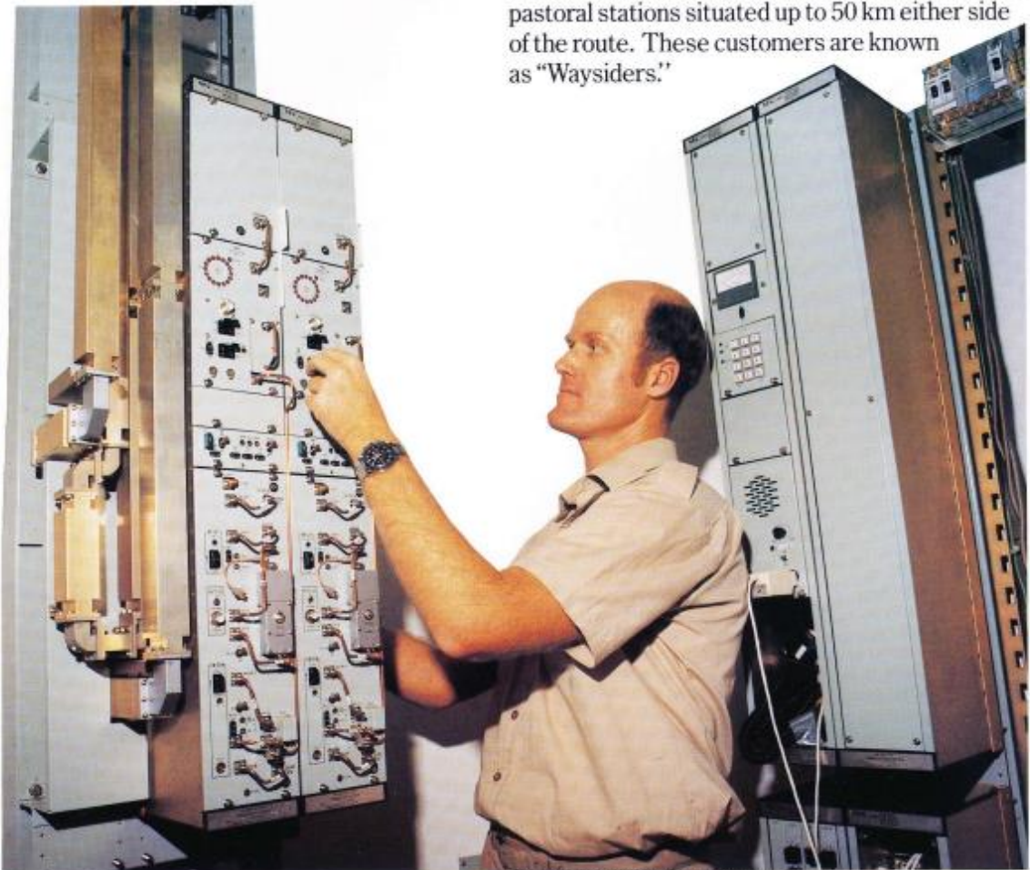
Top left: Section of battery shelter. Above: Checking repeater equipment inside container. Right: Solar panels mounted on shelter.
