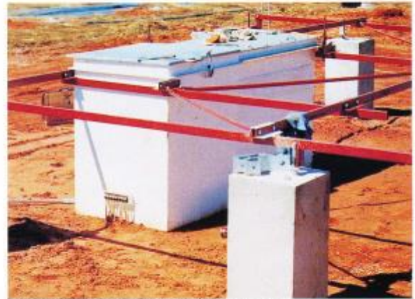
Shelter mounting frame around container entry.
